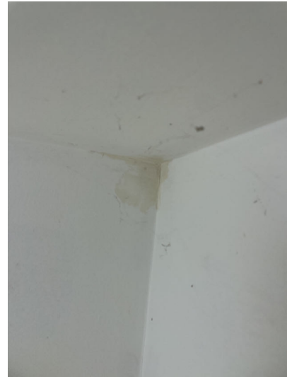
Rear right bedroom: staining
