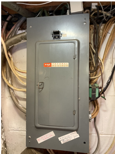
Main panel: Federal Pacific/missing screws
