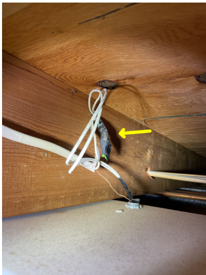
Connection outside junction box/improper wiring
