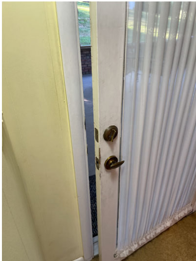
Patio door: does not latch
