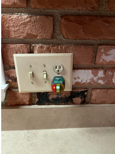
Hot & neutral reversed/not GFCI protected
