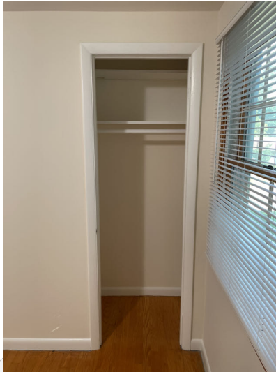
Rear left bedroom: missing door
