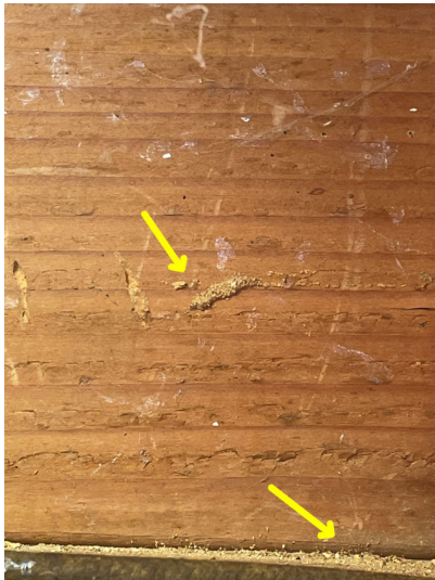
Evidence of WDO
