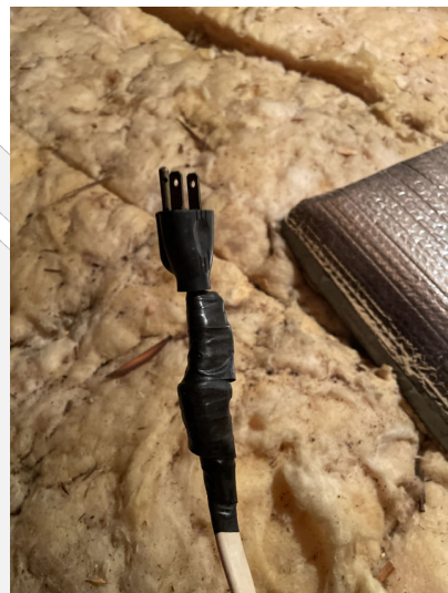
Main attic: Connection outside junction box/improper wiring
