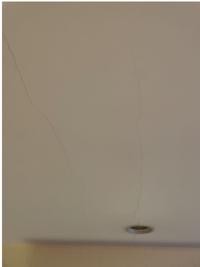
Family room: small crack
