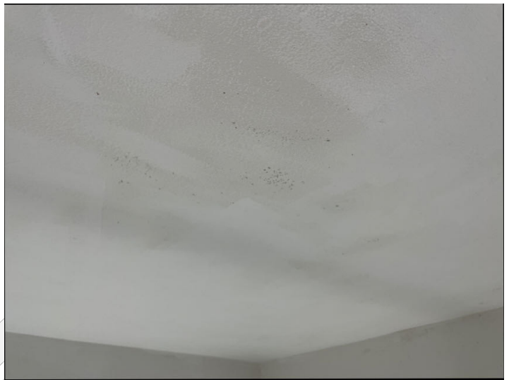
Upstairs hall bath: biological growth
