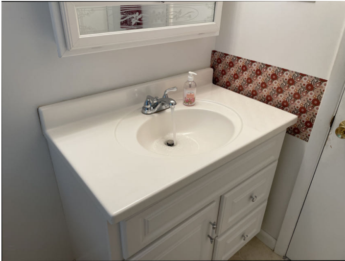
Upstairs hall bath: loose
