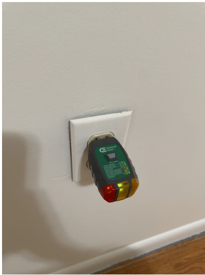
Rear left bedroom: loose/hot & neutral reversed
