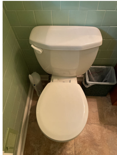
Main floor bath: loose
