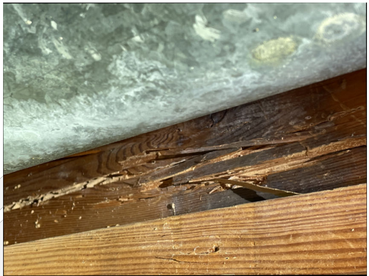
Evidence of WDO
