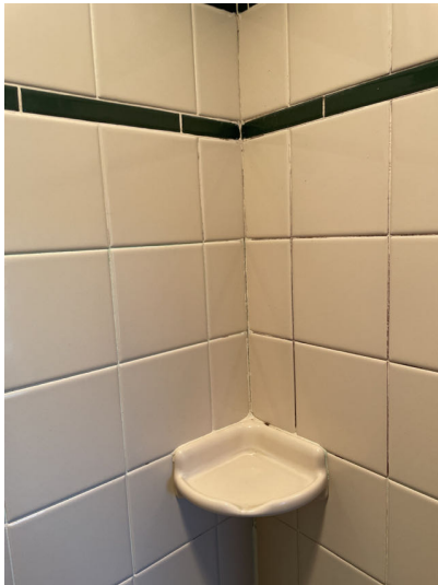
Master bath: damaged grout
