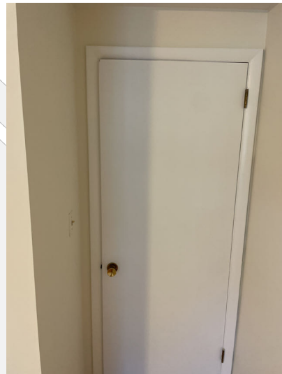
Front left bedroom: rubs framing
