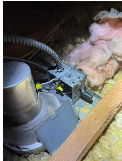
Garage attic: open junction box
