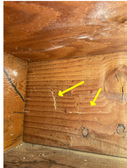
Evidence of WDO
