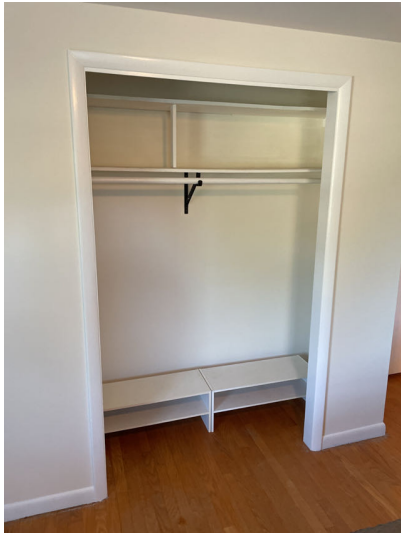
Master bedroom: missing doors
