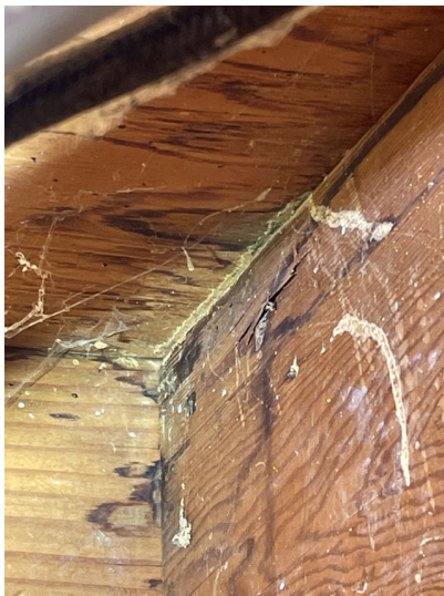
Evidence of WDO
