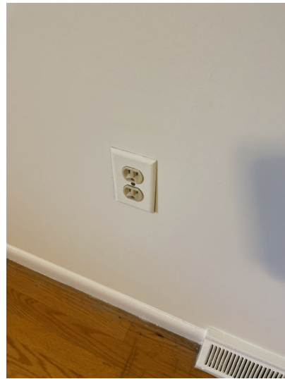
Front left bedroom: loose
