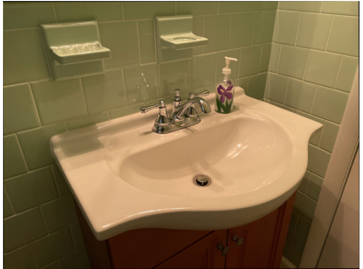
Main floor bath: loose
