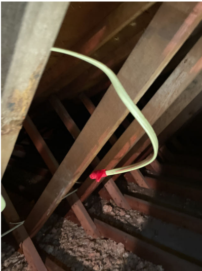
Garage attic: exposed wire
