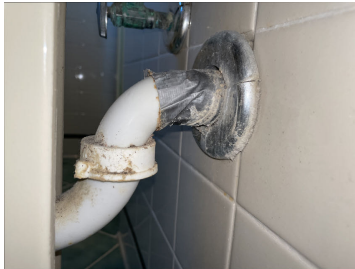
Master bath: unprofessional repair
