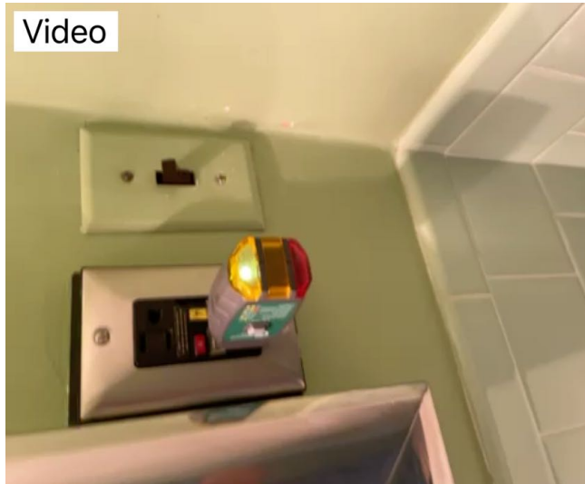
Main floor bath: loose contacts
